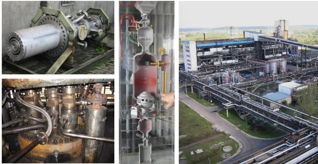
Figure 10: Gasification infrastructure at SVZ Schwarze Pumpe, Germany (2003). Left: Oil-steam burner nozzle and reactor head of entrained flow gasification, middle: model of entrained flow gasifier, right: gasifier building with 6 fixed bed reactors.
