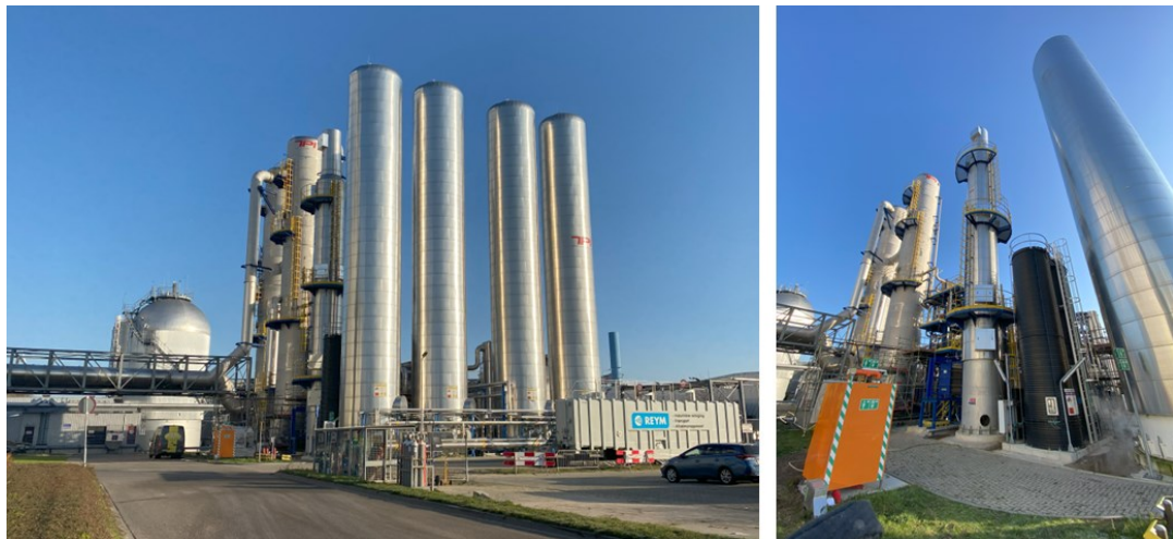
Figure 12: Plant for CO 2 -separation from the flue gas of the MSWI plant Duiven, Netherlands.
